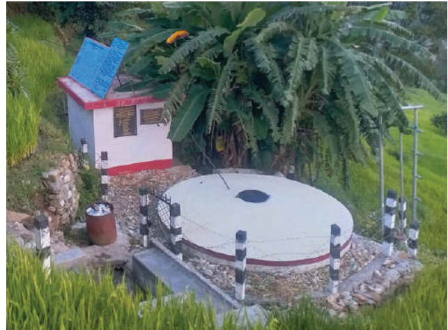
Electric Lifting Water Supply System at Lamgaun, Baglung with sump well and pump house
