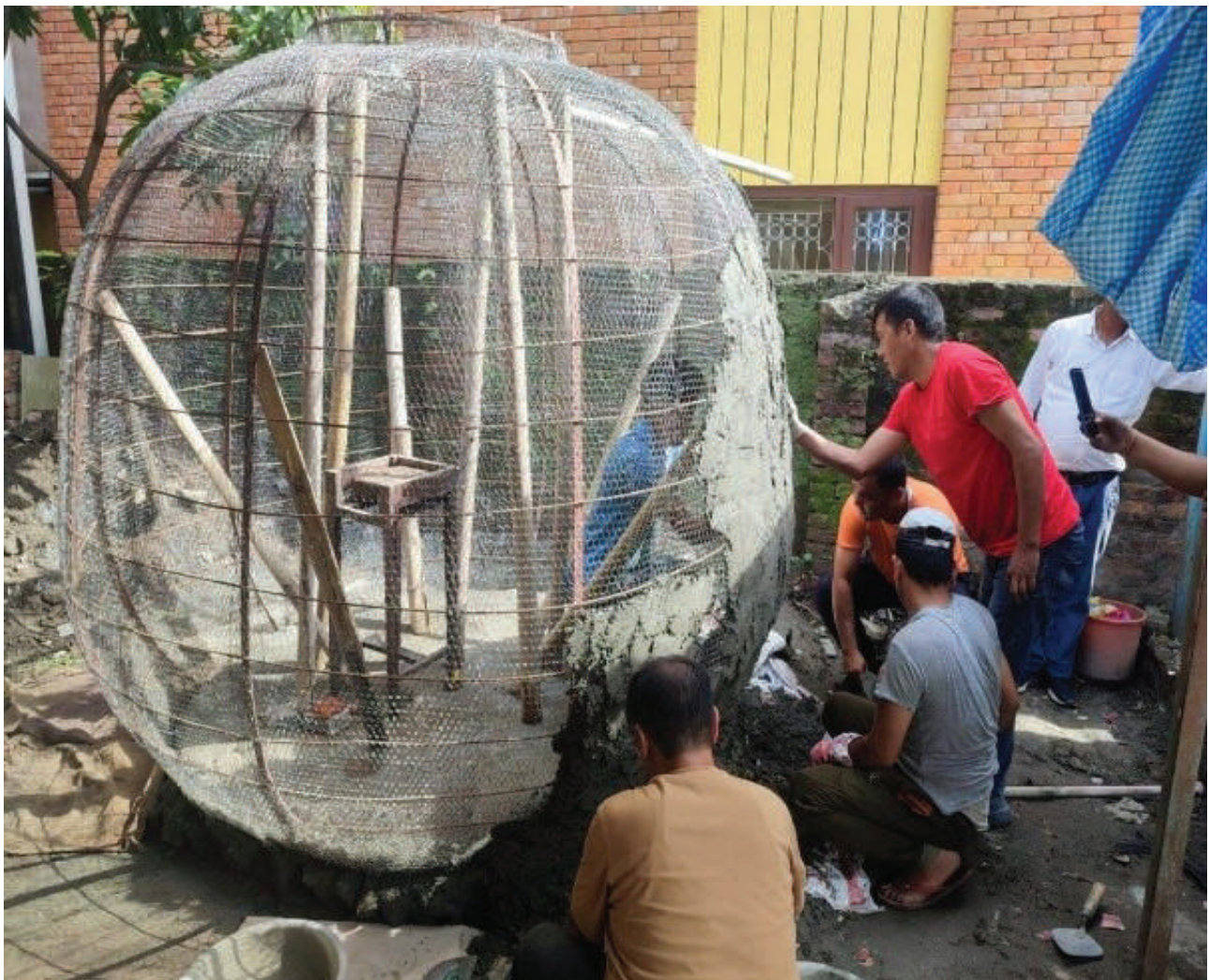
In house Training on construction of Rain water Harvesting Pumpkin Tank at NEWAH HQ
