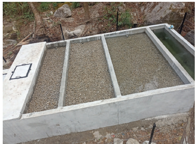
Roughing Filter, Sindhuli
